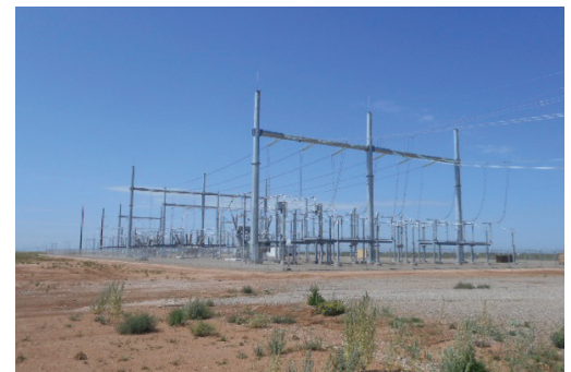
Xcel Energy built the Crossroads Substation outside of Portales to interconnect the new 250 MW Roosevelt Wind Farm.
